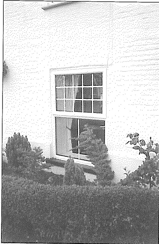
A replacement PVCu window; note the over-thick frames, and the glazing beads which are set between the two panes of the double glazing.
