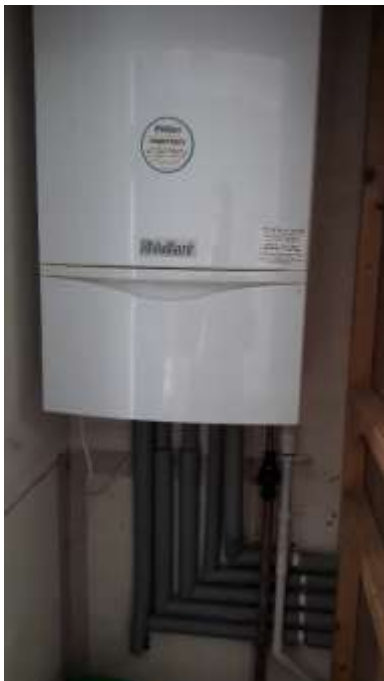
Figure 5: Natural Gas Combi Boiler Located in 1 st Floor Cupboard
