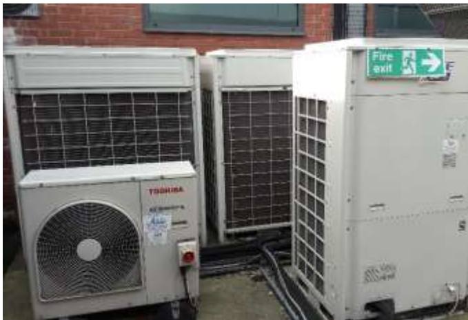
Figure 6: The Dry Sports Centre HVAC Inverters Located in the Central Yard
