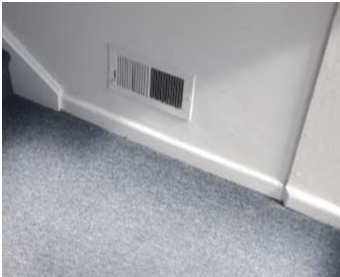
Figure 2: Cavity Air Vent Located at the Foot of the Staircase in the Hall
