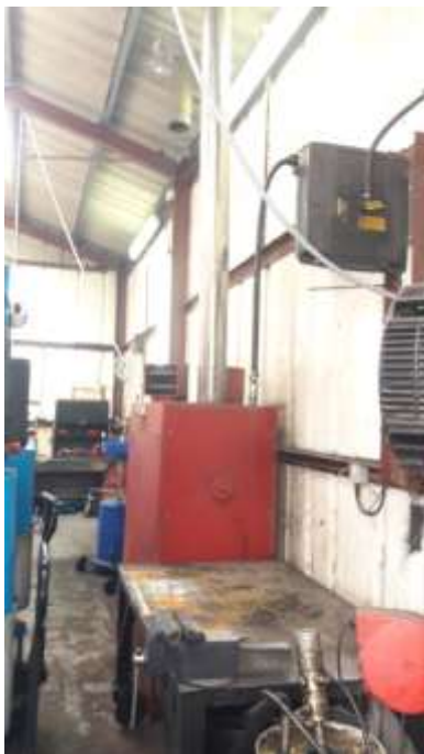
Figure 6: One of Two Existing Oil Heaters in the Smaller Workshops
