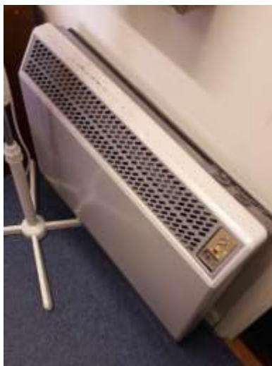
Figure 9: Storage Heater in the Reception Office.
