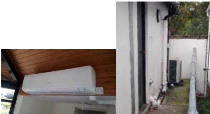
Figure 7: Internal and External Elements of the HVAC Supplying the Octagonal room
