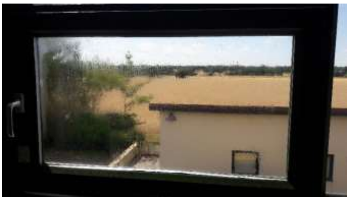
Figure 7: An Example of the Broken-Down Double-Glazing Units in the Main Building.
