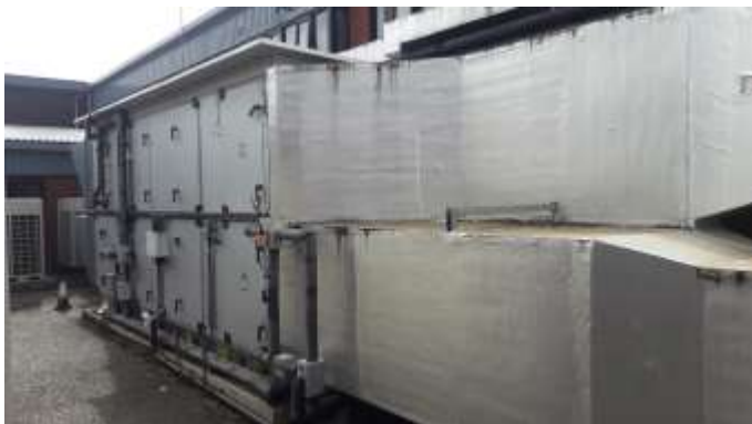
Figure 7: Air Handling Unit for the Dry Fitness Centre.
