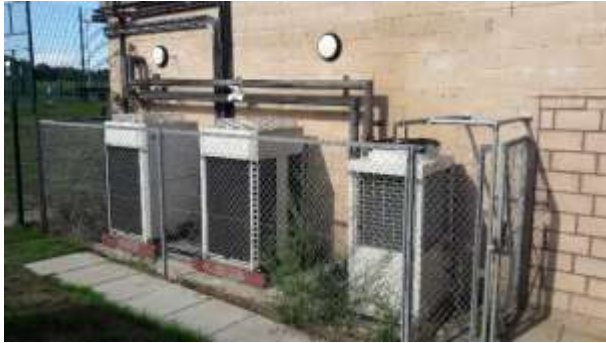
Figure 4: HVAC Condenser Units Supplying Space Heating
