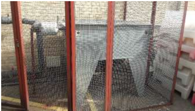
Figure 5: The CHP External Water Radiator and Fan Assembly
