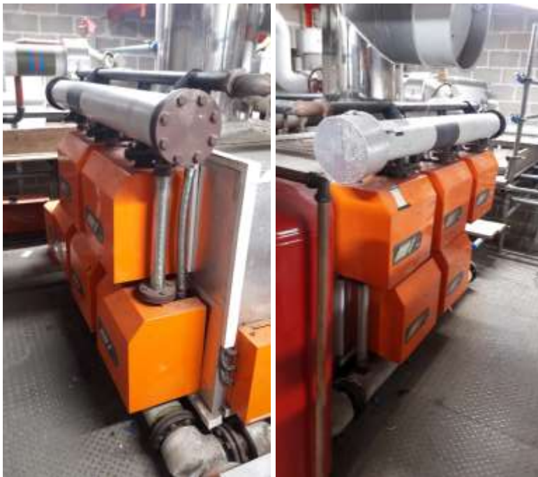
Figure 6: The Pool Natural Gas Heating System
