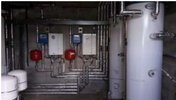
Figure 5: Twin Calorifiers and Water Storage Vessels
