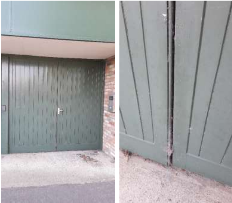
Figure 6: Poorly Fitting Wood Barn Doors Leading Directly into Unit 27.
