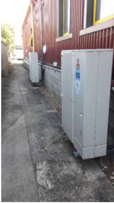
Figure 5: The Gym HVAC Systems
