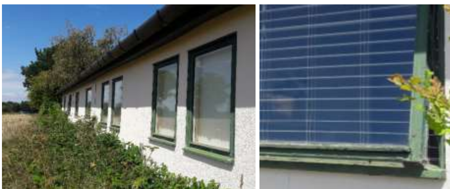
Figure 8: Poorly Fitting Wooden Windows in The Annexe.
