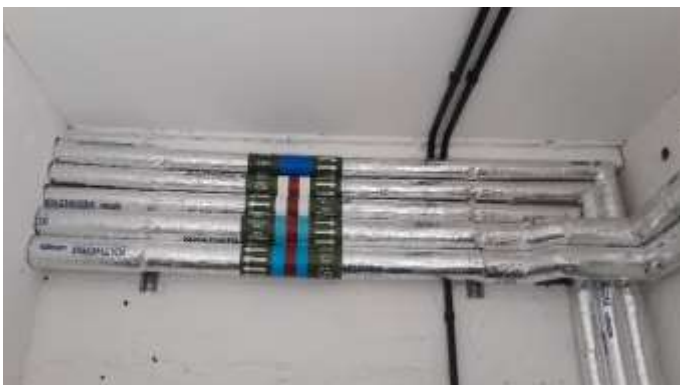
Figure 5: Part of the Ground Sourced Heat Pump Distribution System
