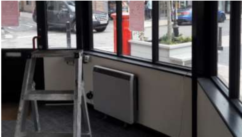
Figure 6: One of Two Storage Heaters Located in the Octagonal Room
