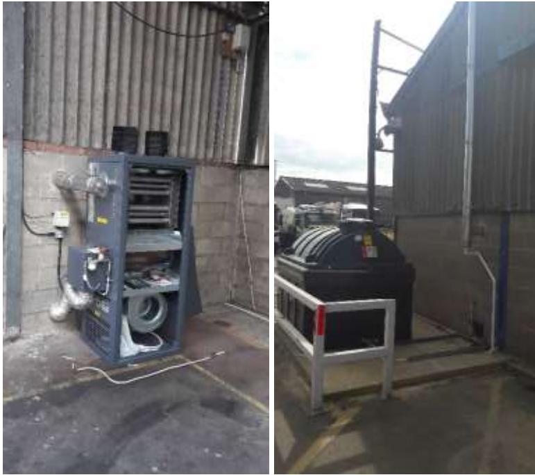
Figure 7: New Oil Heater and Storage Tank at the Large Workshop
