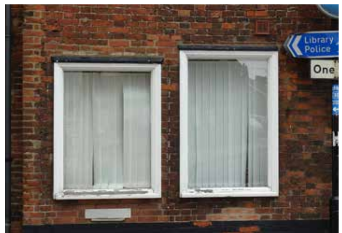
Unsuitable window design
