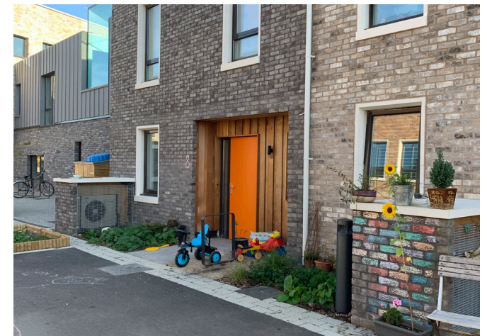
Heat pumps are carefully integrated in front of homes at this development on Marmalade Lane, Cambridge.
