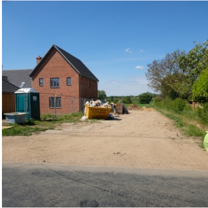
Figure 35: Photograph of the development showing Gap B.
